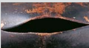
FREEZE RUPTURE Caused by low water flow in the evaporator.
