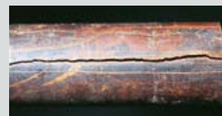
STRESS CRACKING Longitudinal or intergranular cracks caused by high water flow.
