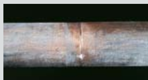
TUBE SUPPORT WEAR Caused by the tube/support contact. Although this phenomenon is quite rare, it must be quickly detected.
