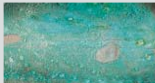
DEPOSIT CORROSION Deposits of algae and slime caused by inadequate water treatment.
