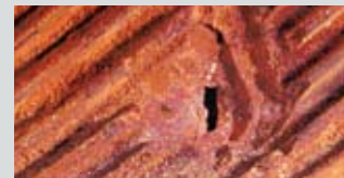
INTERNAL PITTING Caused by an abnormal presence of aggressive elements in water.
