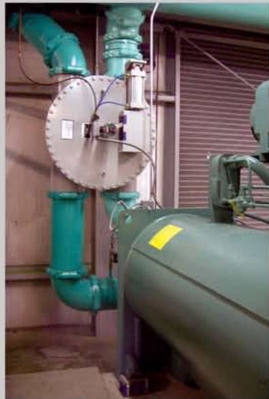
The ATB System 4-way valve reverses the condenser water flow for about 30 seconds every 6 hours.
